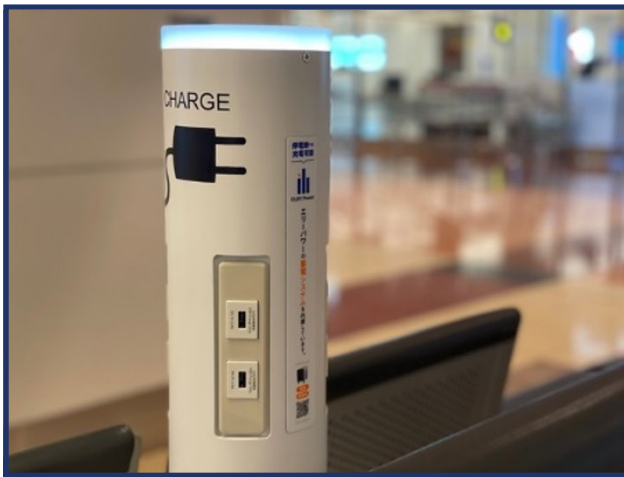
Figure 9 USB charging port installed at Haneda Airport [*]35
